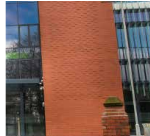
Contemporary precedent of brickwork detailing - Individual projecting bricks to create textural panel
